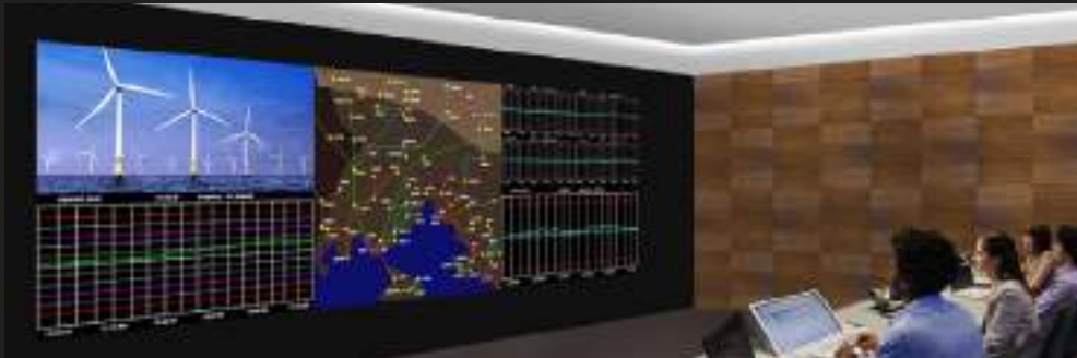
Control / command rooms
