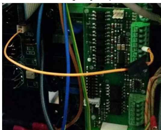
Emergency stop enabled
